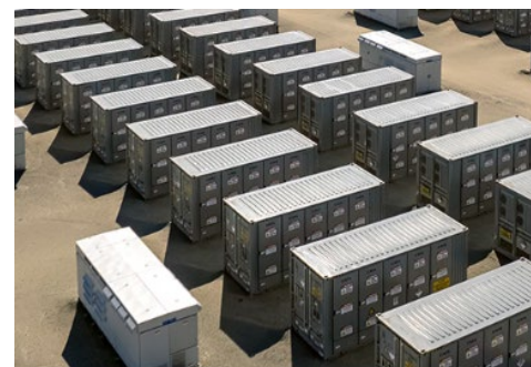
50MW Battery Storage, Georgia
