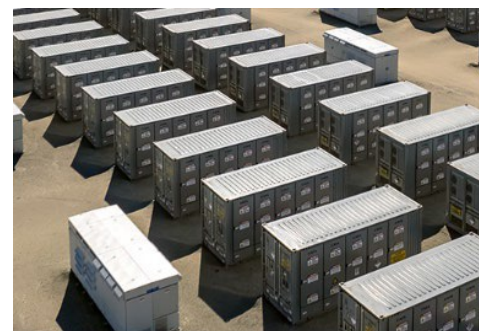
50MW Battery Storage, Georgia
